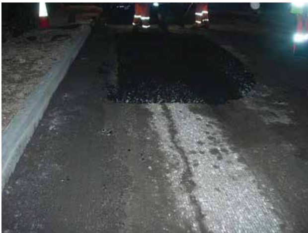
View of the planed/damaged surface
